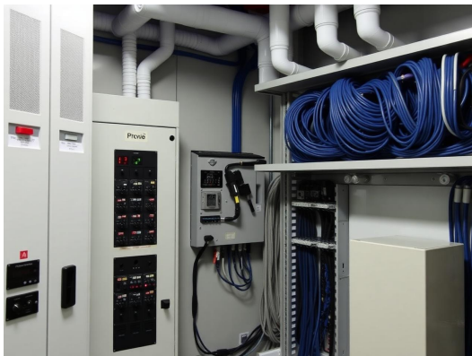
Electrical & control panels
